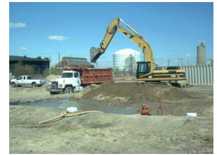
A view of the loading of petroleum contaminated soil into a dump truck for disposal
